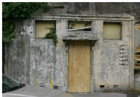
Condition 5 (very poor)
